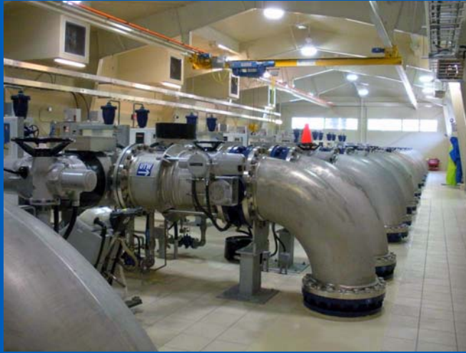
Victoria, British Columbia, Canada – 150 mgd UV treatment system
