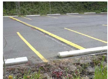
Berm (Speed bump) across parking lot to divert runoff into the swale; September 2002
