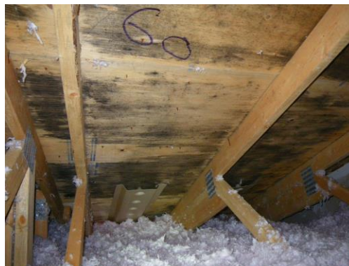
Figure 14: North facing attic roof sheathing for same attic as Figure 13 showing significant fungal growth
