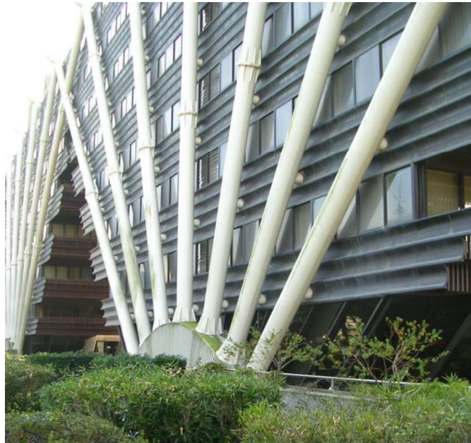
Figure 2 - Fire Protected External Steelwork. Project: Torri Esso – Rome, Architect: Julio Lafuente. Photo Courtesy Of Etex Group.
