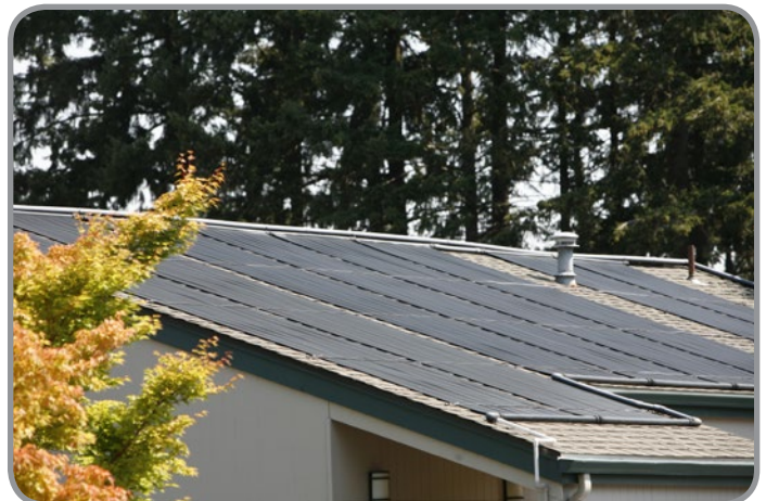
Solar pool heating
