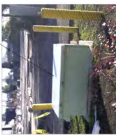
EXISTING TELECOM VAULT ACCESS
