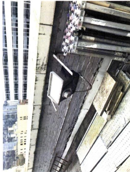
EXISTING CLOCK UPLIGHTS: PHOSPHOR-COATED MERCURY VAPOR 250W. NOTE FIXTURE IS NOT VISIBLE TO PUBLIC.
