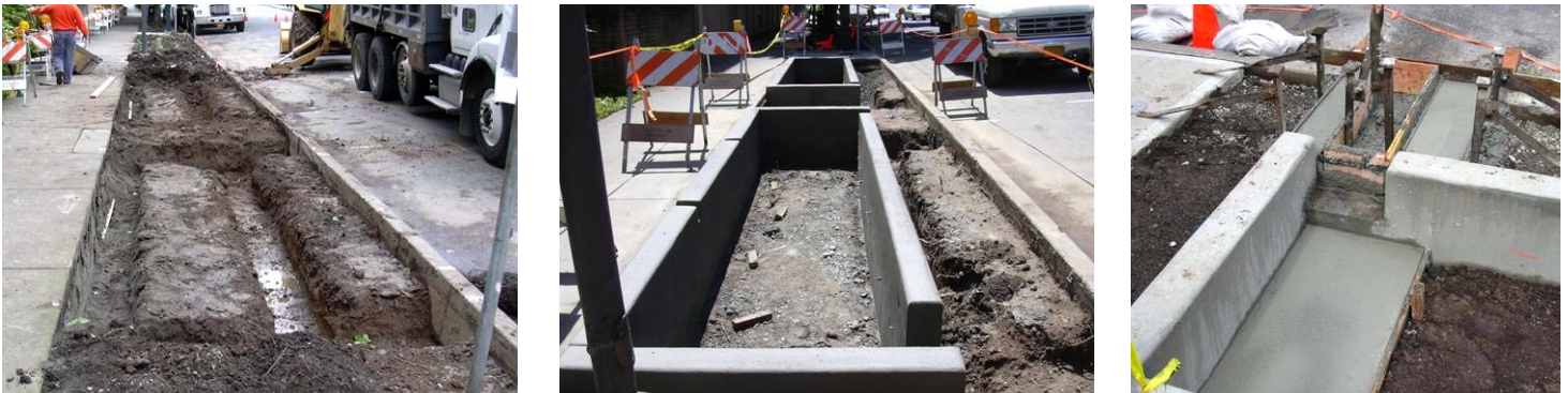
Stormwater Street Planters under construction: Grading (far left); Formed concrete walls (center); Forming the concrete trench and sediment collection pad (far right)
