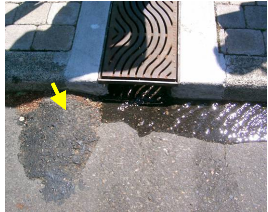
Asphalt berm at facility inlet to help direct stormwater flow into the stormwater planter
