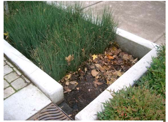
Sediment collecting behind the juncus on the concrete pad
