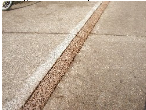
Figure 6: Porous asphalt radials
