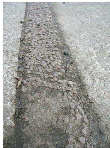
Figure 10: Porous asphalt clogged with debris
