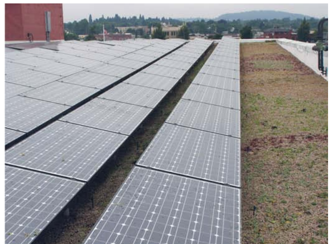
International Harvester Building Eco Roof- After - upon construction completion date July 2010
