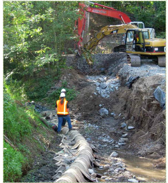
Removal of decommissioned CSO pipe with streambank restoration at Stephens Creek confluence.
