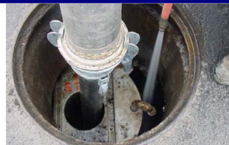
Figure 5 – Vacuuming Sediment Sump
