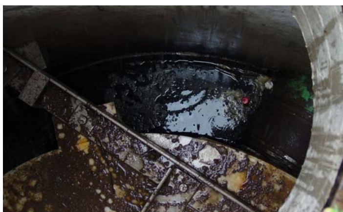
Figure 7: View of outer annulus of floatables and oil collection zone
