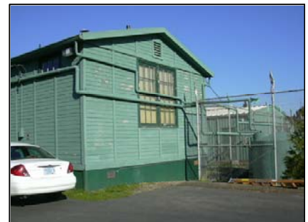
Classroom from which runoff for the three classrooms drains to the cisterns - note aerial pipes
