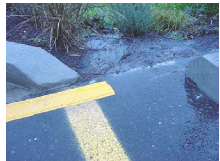
Raised parking stripe directing runoff into the swale; November 2000.
