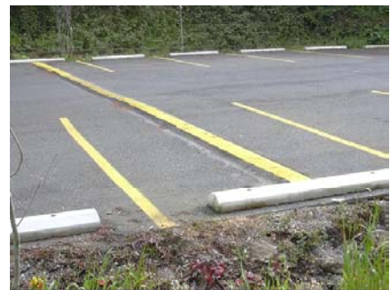
Berm (Speed bump) across parking lot to divert runoff into the swale; September 2002
