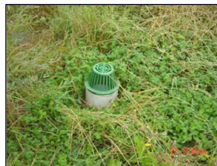
Standpipe overflow in the last compartment of the swale
