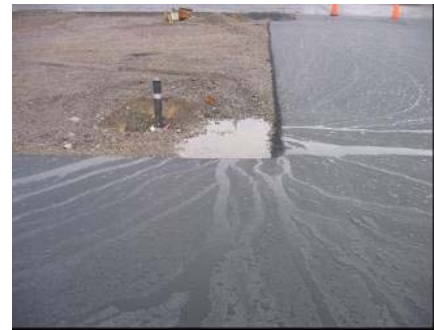
Flow paths draining to the location of the landscape infiltration basin (yet to be built); 2002
