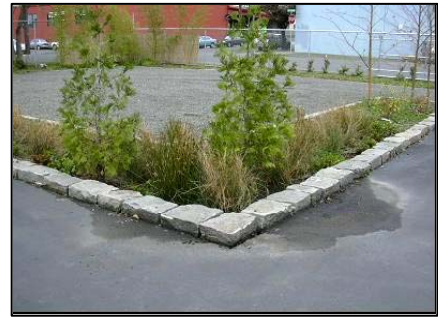
Landscape infiltration basin after a storm, 2003. Note damp pavement where runoff recently ponded on asphalt surface.
