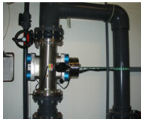
Portland Parks & Recreation has installed UV filters on all Portland City indoor pools.
