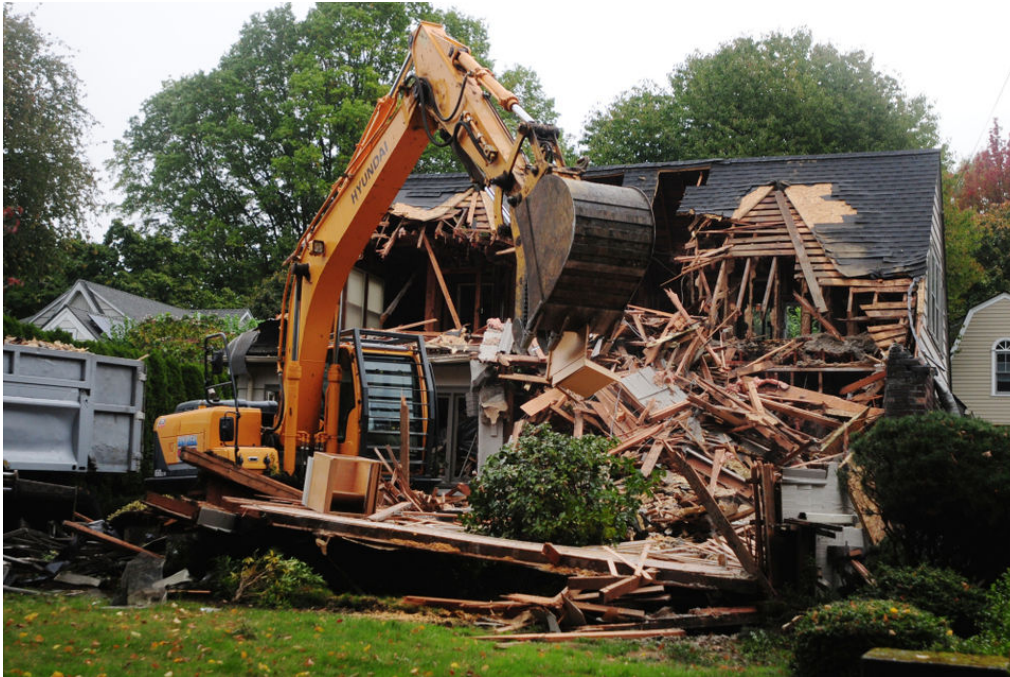
A house in Southeast Portland's Eastmoreland neighborhood is demolished on Monday, Oct. 20, 2014. (Mark Graves/The Oregonian)
