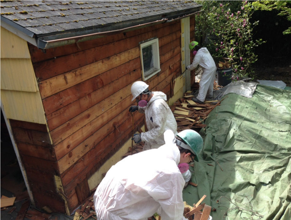
A crew from Lovett Deconstruction disassembles a Southeast Portland house by hand in Portland on April 14, 2015. The city mandated deconstruction for historic homes, which also served to minimize toxic dust, but advocates argued the policy offered public health benefits mostly to well-off neighborhoods. (Mike Francis/Staff)
