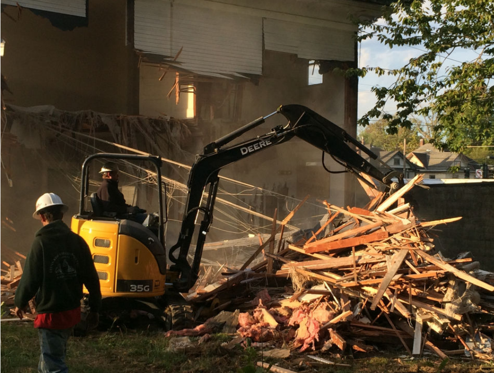
Work crews demolished a house on Southeast Hawthorne Boulevard on October 16, 2015. New city rules requiring the control of dust and debris took effect in July 2018. (Stuart Tomlinson/Staff)
