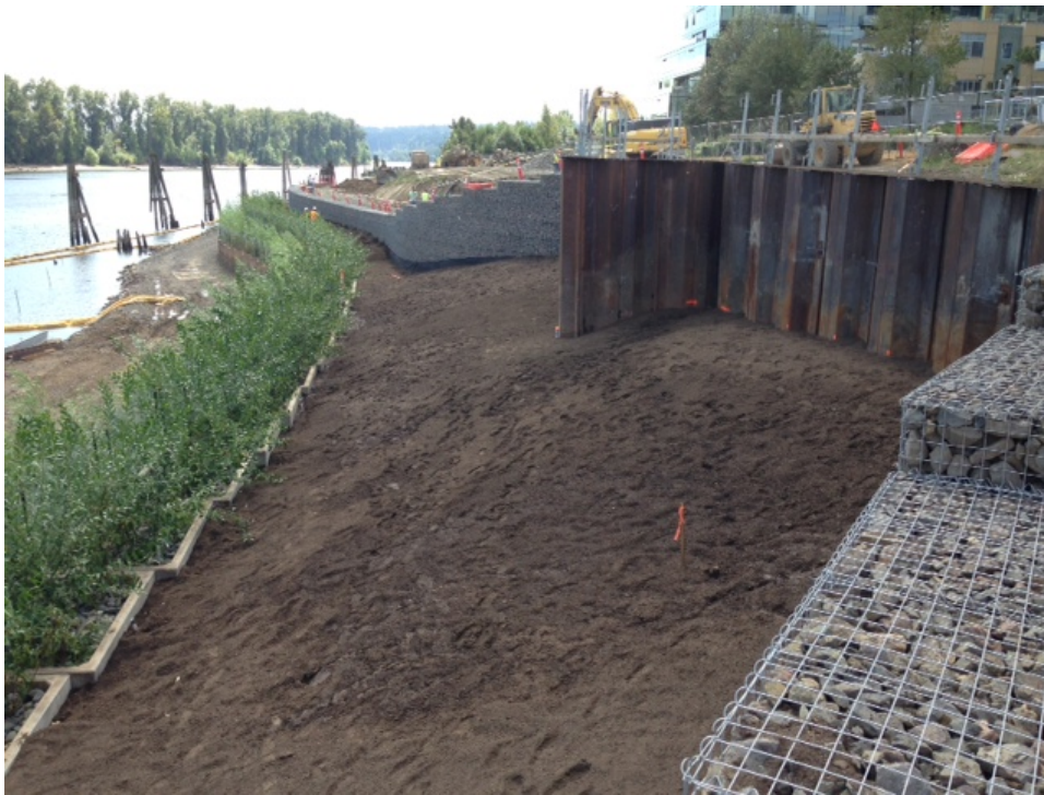
At left, shallow water habitat and vault wall with willows; at right, wire gabion wall and tall sheet pile wall; at center, new planting bed for native vegetation.
