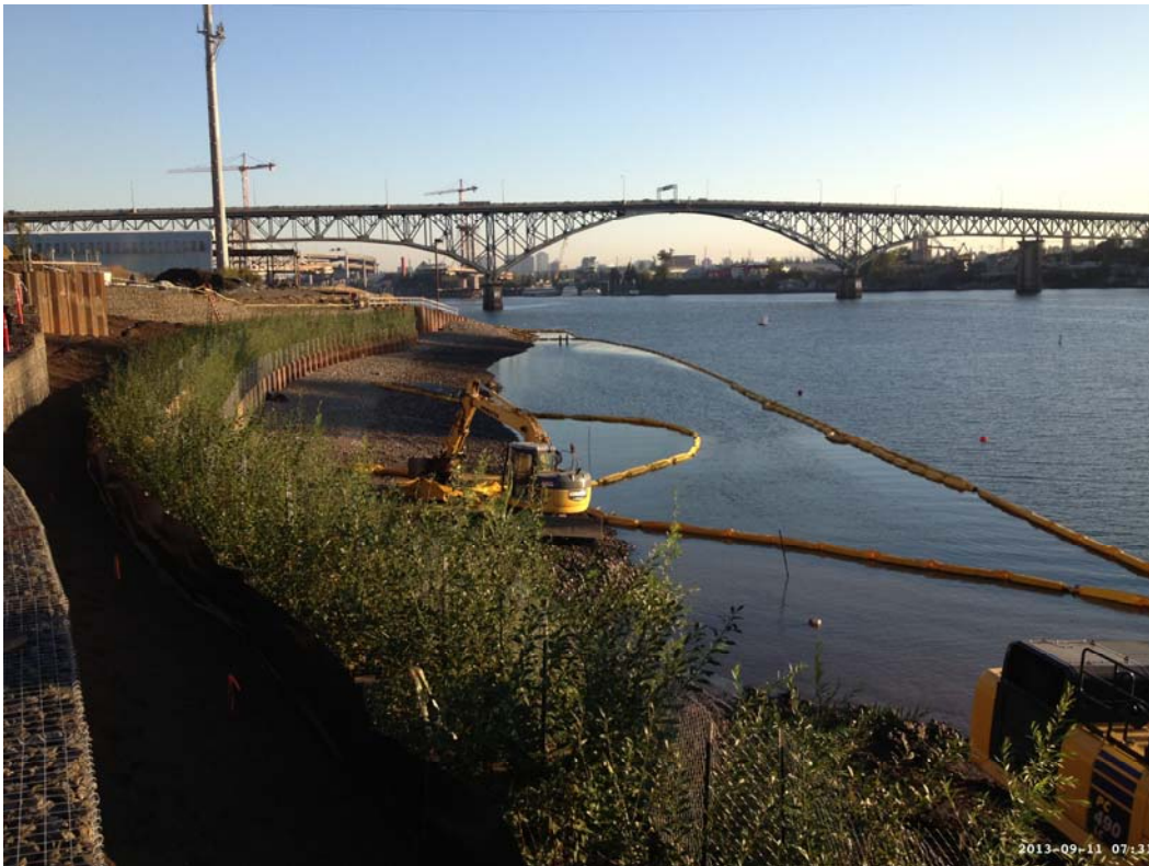
At upper left, the Curry St. sheetpile wall; at center, the vault wall with willows; at right, the shallow water habitat and yellow sediment curtains.
