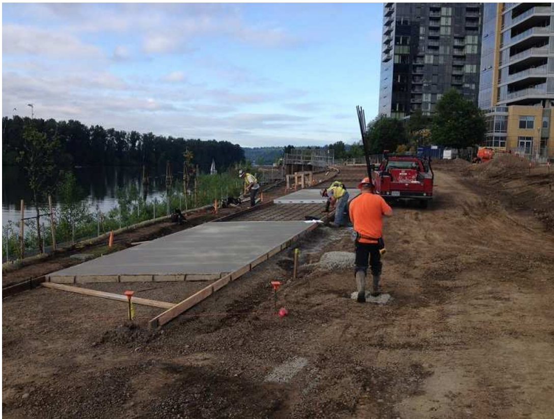
Looking south from near Whittaker: JW Fowler Co. employees build a section the pedestrian path near the Curry Street overlook. At left, greenery from the reconstructed riverbank can be seen.
