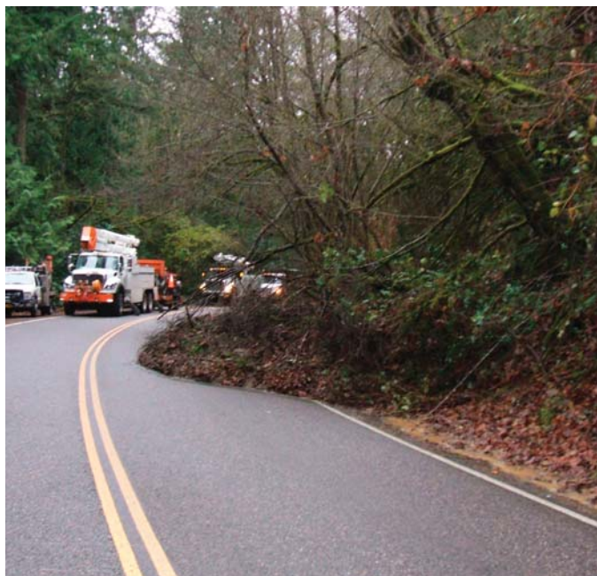
A landslide occurred on NW Cornell just west of NW 53rd Drive. The Urban Forestry crew removed two 16" diameter alder trees that came down with the mud. The 55' high trees were only a few feet from high voltage lines and PGE assisted with power shut off and road closures.
